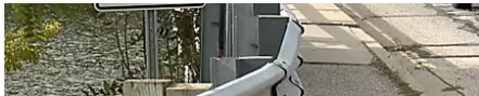
'Everybody was feeling very good': Funding pulled for aging Smith's Bridge in Ferrysburg FOX 17 West Michigan News
